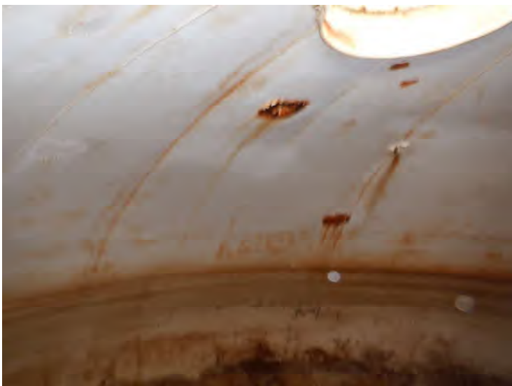
51) Coating failures on the wet interior roof.
