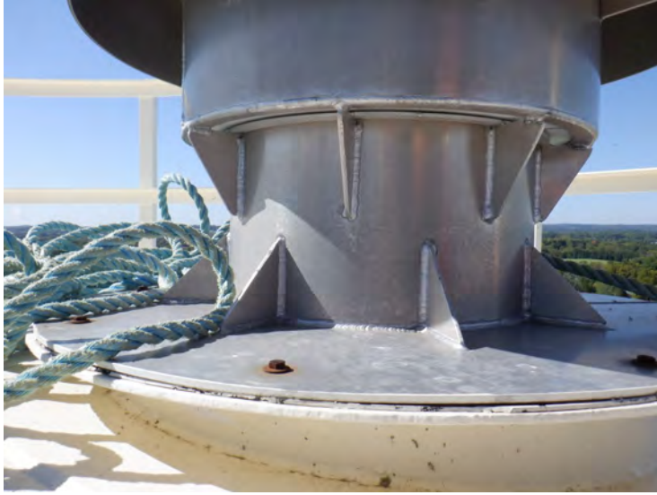
22) The roof vent pressure plate was properly aligned and free to move.
