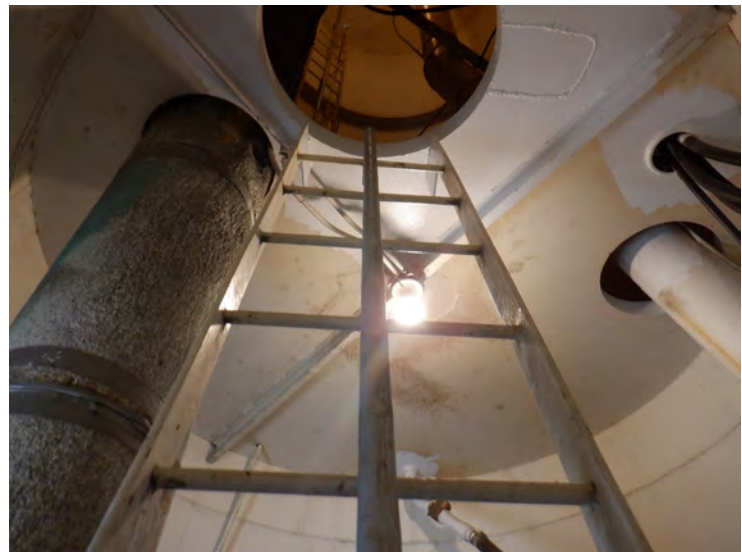
29) The baseball ladder is in good condition. The ladder is equipped with a fall prevention device.
