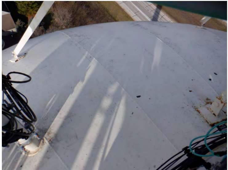
20) Coating failures on the roof.
