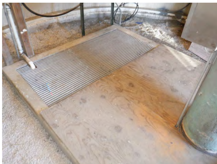
66) The cover over the pit in the baseball is in good condition.
