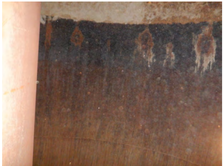
53) There is heavy mineral staining on the wet interior sidewall but no coating failures.
