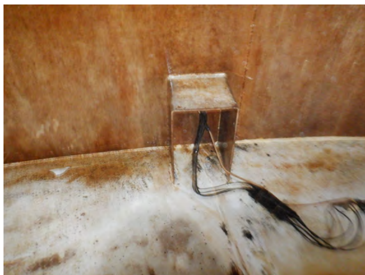
54) The cathodic protection pressure fitting has a deflector plate around it.
