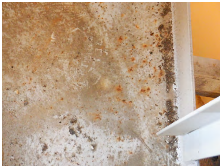
39) Minor coating failures on the top platform.
