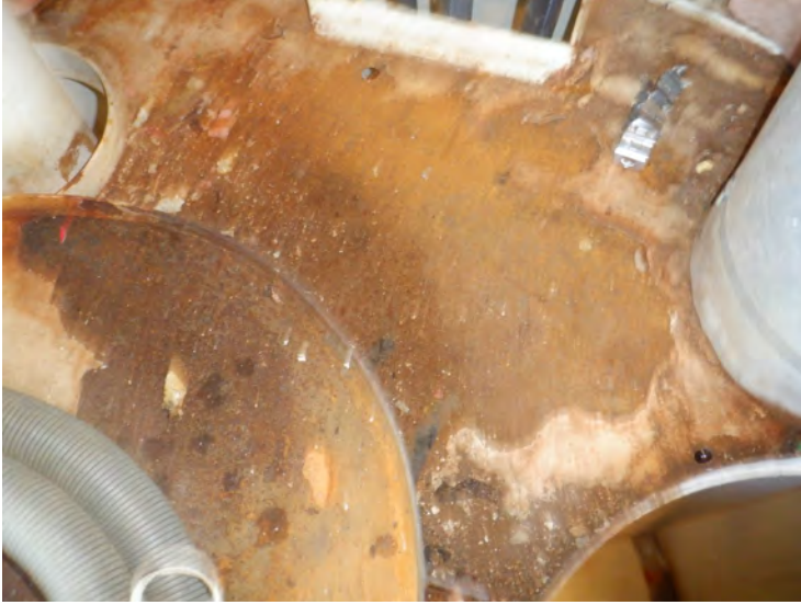
43) Coating failure on the top platform.
