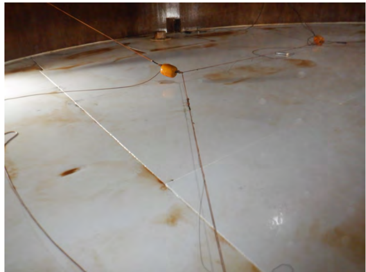
59) The cathodic protection system appears to be in good condition.
