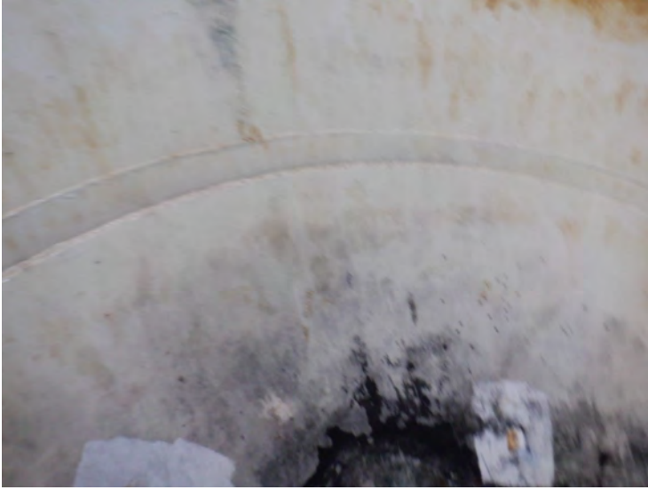
61) The coating on the bowl is in good condition overall.
