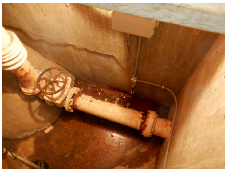
66) Coating failures on the pit piping.
