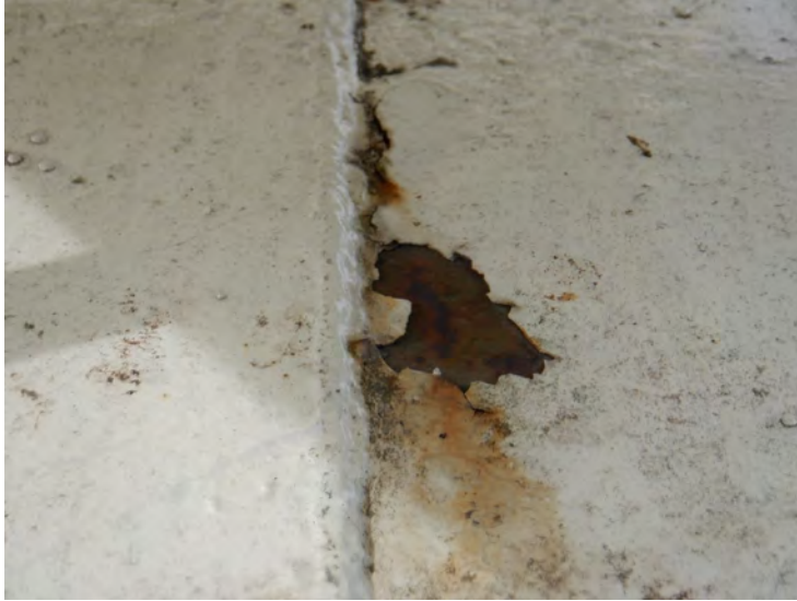
22) Spot coating failures on the roof.
