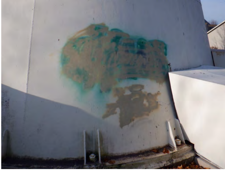
7) Coating failures on the basebell.
