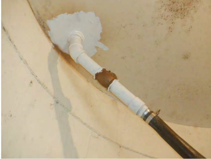
28) There is a check valve on the condensate platform drain.
