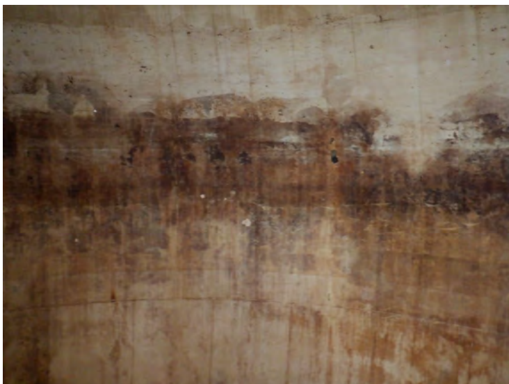
54) The wet interior sidewall coating is in poor condition overall.
