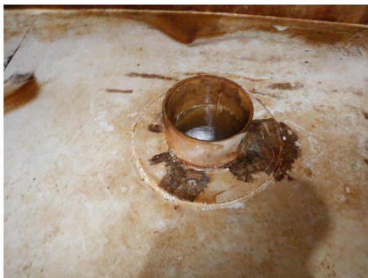
60) The fill/draw pipe is in good condition. There is not a deflector plate or bar over the top of the pipe.
