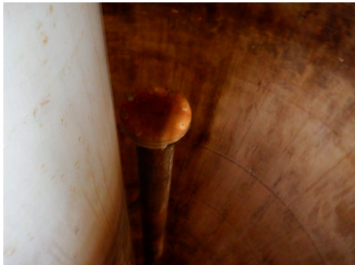
56) There is an abandoned pipe with a blind flange in the wet interior that extends up near the high-water level.
