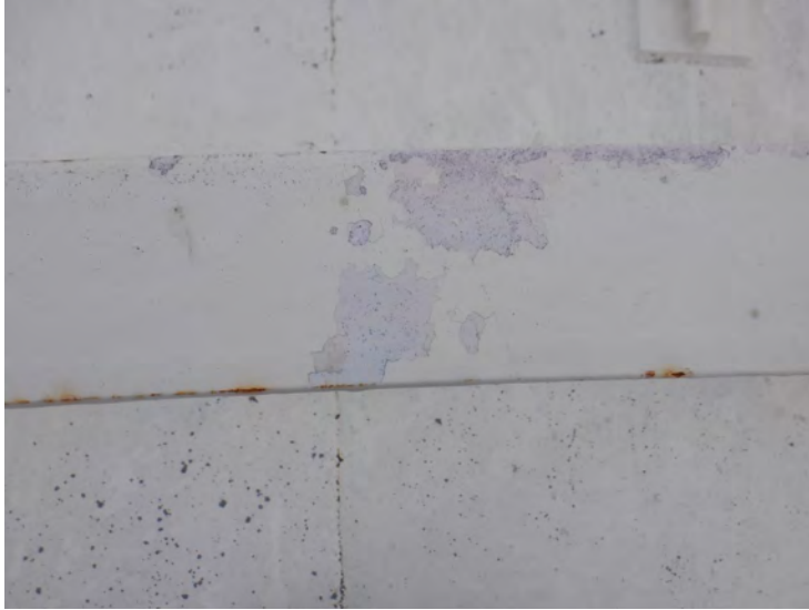
28) There is delamination along the handrail.
