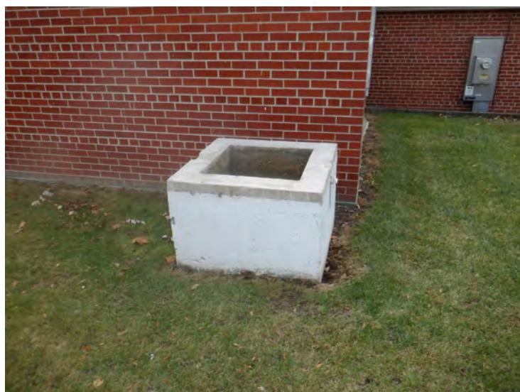
6) The roof hatch curb is more than 24 inches above grade.
