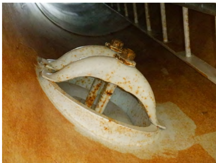
48) Coating failures on the wet interior manway.
