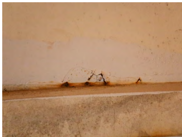
33) Coating failures along a stiffener in the dry riser.
