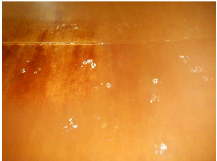
50) There are blisters in the sidewall coating on the lower sidewall panels.
