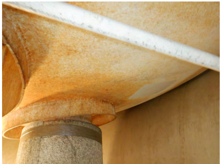
44) Extensive rust bleedthrough on the bowl.
