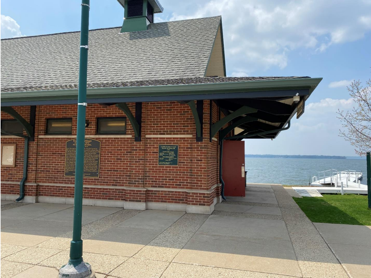
Lakefront Park, photos in order of NE, NW, SW, SE around building. Open air portion is the south/southeast portion of structure.
