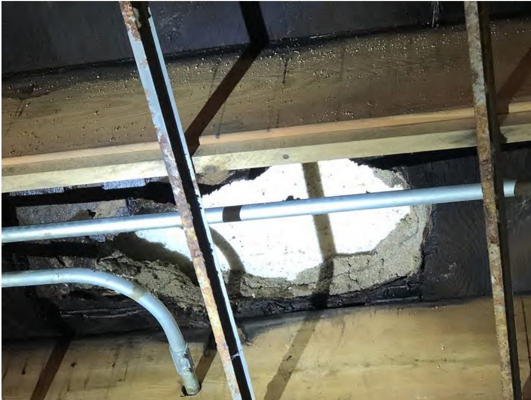
Area of missing decking
