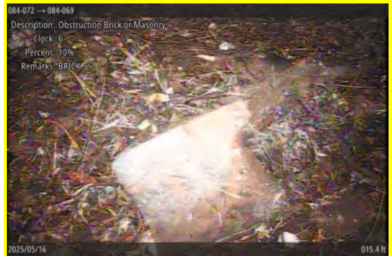
[Grade 2] Obstruction Brick or Masonry at 015.4 ft, 6 o'clock | BRICK
