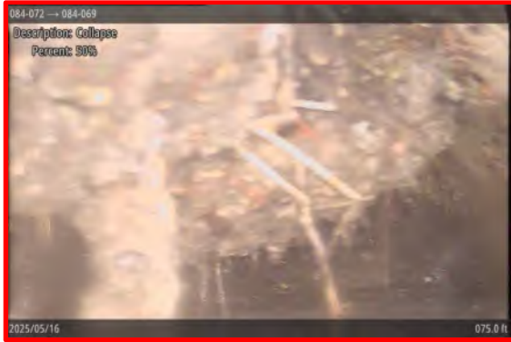
[Grade 5] Collapse at 075.0 ft
