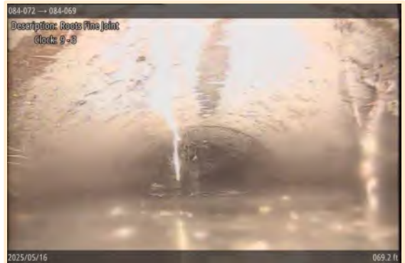
[Grade 1] Roots Fine Joint at 069.3 ft, 9 - 3 o'clock
