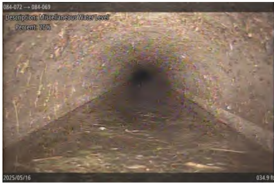
Miscellaneous Water Level at 034.9 ft
