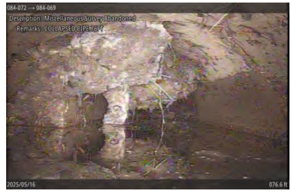
Miscellaneous Survey Abandoned at 076.6 ft | COLLAPSED PIPE 76FT
