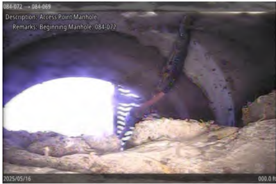
Access Point Manhole at 000.0 ft | Beginning Manhole: 084-072
