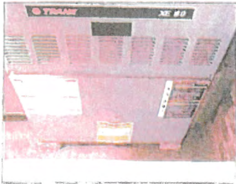
27. TRANE gas fired furnices (2)
