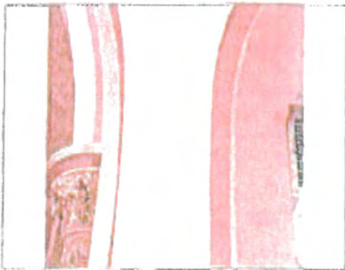
17. Typical of cracks in plaster.
