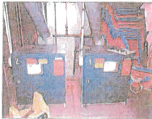
24. Mechanical room, twin Vaillant boilers.
