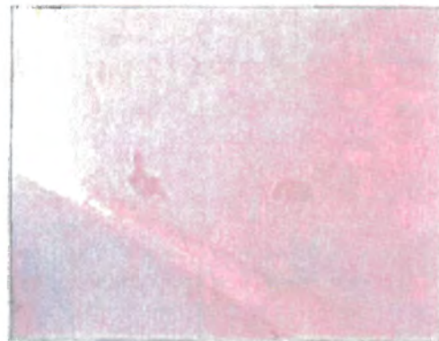
18. Typical of paint peeling from plaster surface
