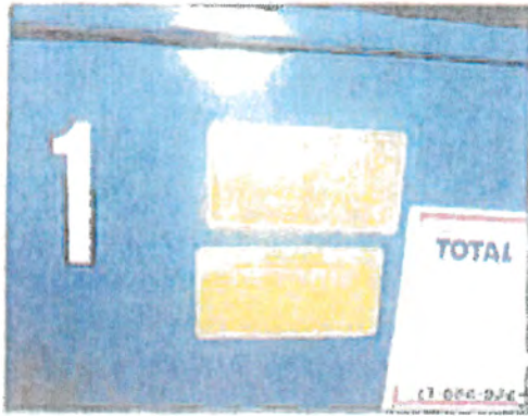
25. Boiler #1 inspection date
